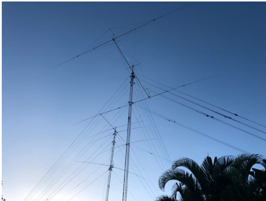
oben: 2 Element 80m Yagi (Montage mittels Helikopter), dahinter 4 Element full-size 40m Beam und 40m Dipol darunter
